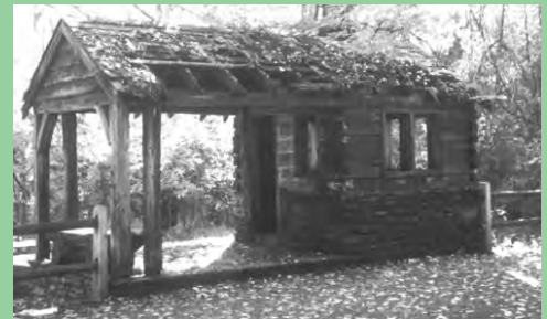
Allen's Lane Guard Shelter in disrepair (1996), the first WPA shelter in Wissahickon Valley Park to be surveyed and restored.
