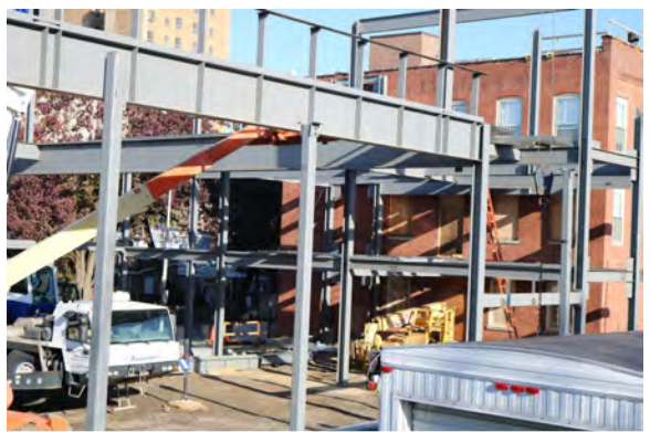
Greene Street Friends School campus expansion under construction, view along Armat Street in fall of 2017. Image: greenestreetfriends.org
