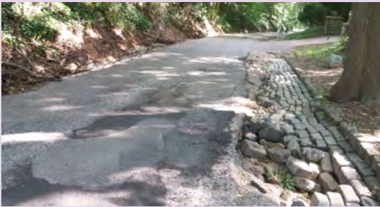
Many Wissahickon Park access streets cannot safely accommodate the variety of users that visit the park. View of the deteriorating conditions of Kitchens Lane near Wissahickon Avenue.
