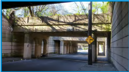
View of abandoned rail spurs over Armat Street show their potential for reuse as pedestrian circulation and park space.
